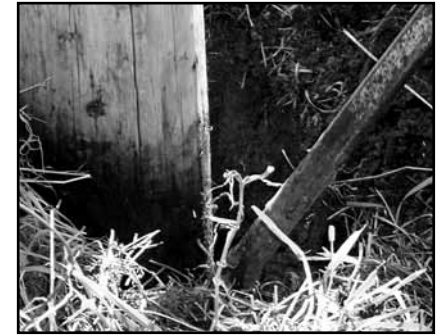
The base on this pole is being treated to extend the life of the pole.
