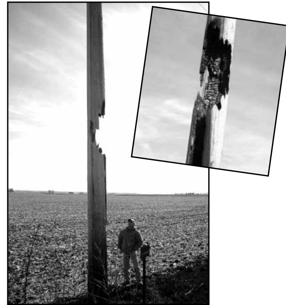
A NIPCO lineman examines a fire-damaged pole on the Clay Substation tap line near Modale in Harrison County. The burned pole was replaced with a steel pole.
